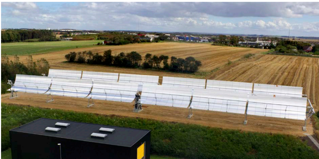
Figure 1. Overview picture of the Aalborg CSP plant in Thisted.
