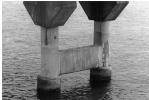
Figure 6.5: Spalling at pier of Florida Keys Bridges, FL, USA, due to corrosion of the epoxy-coated reinforcement. From [COWI, 2007c].
